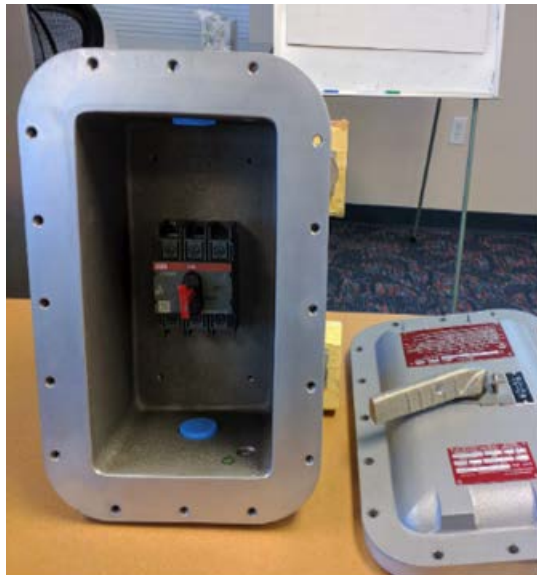
Figure 2 - Enclosure with ABB Disconnect Installed
